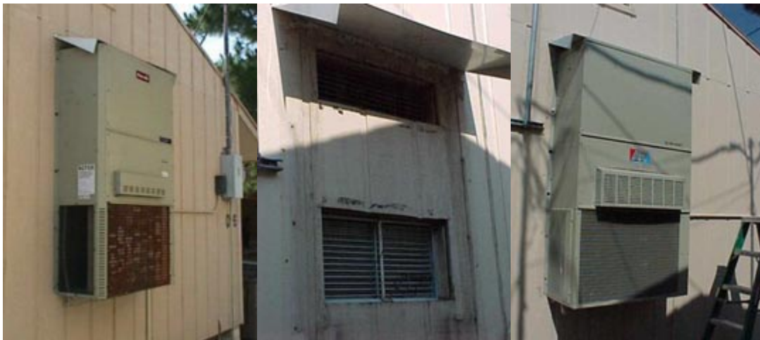
Figure 17. Left: old unit; Center: outer unit removed showing thru-the-wall return grill and supply duct; Right: new HVAC unit.
