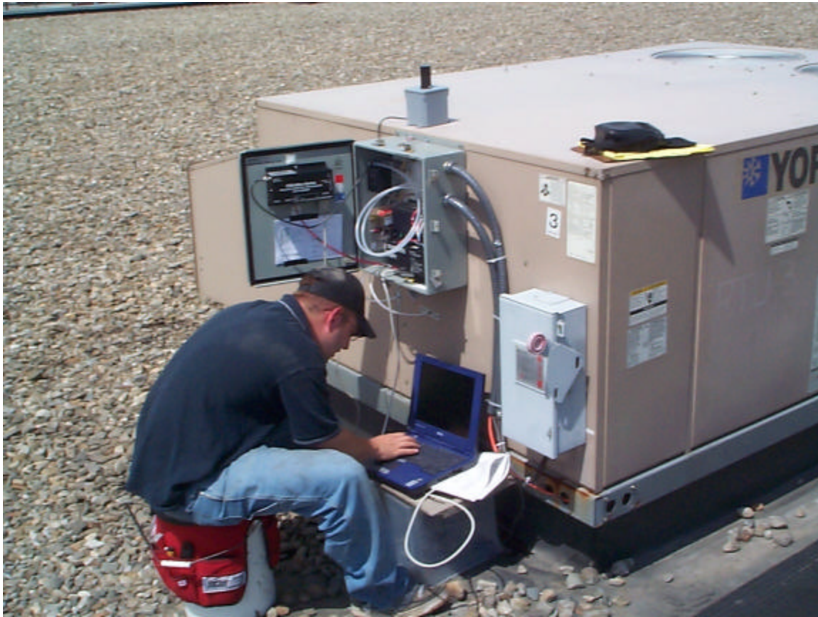
Figure 1. RTU With DAS System Installed
