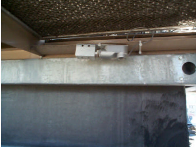
Figure 11. Ambient Temperature Sensor Under Fresh Air Intake
