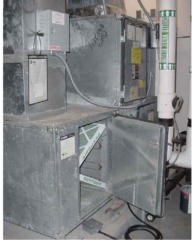
Figure 4-2. Commercial Air Handler (Site 7)
