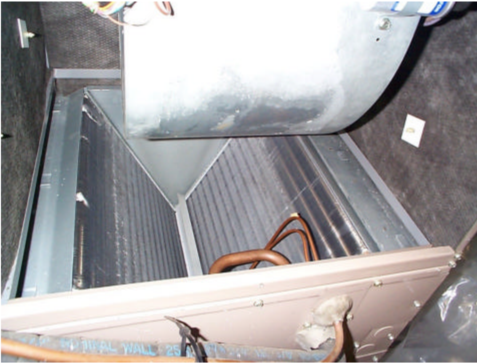
Figure 11. Coil in AHU #2
