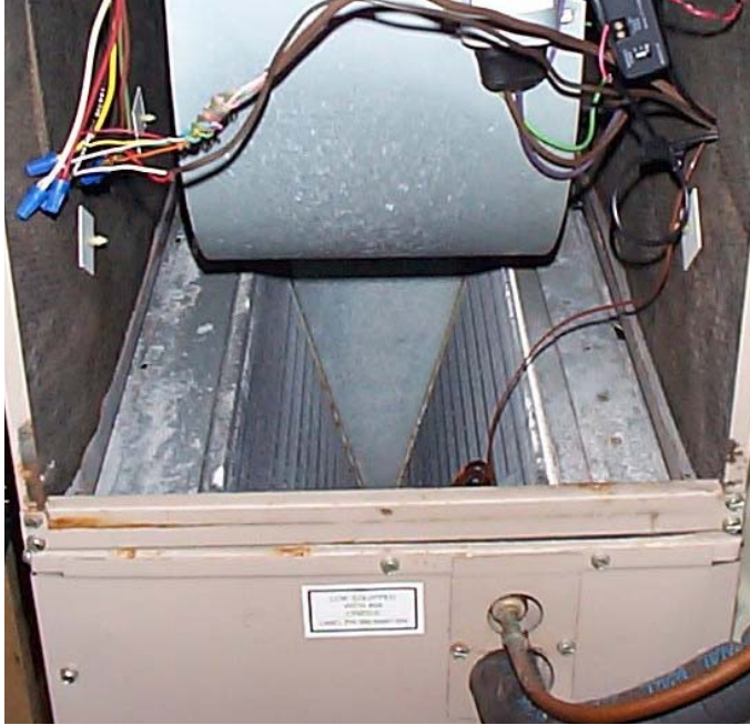
Figure 4-1. Residential Air Handler (Site 1, 2 nd Floor Unit)
