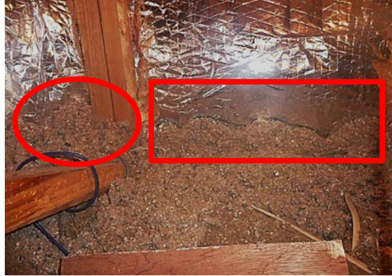
Figure 6. Duct section PA after insulation wrap has been installed. In the red rectangle, the foil facing will be tucked under and cellulose added. In the red circle, the foil facing has been tucked under, and a small amount of cellulose insulation has been added where the duct wrap meets the existing cellulose.
