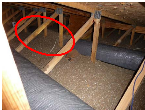
Figure 4. Flex duct section 8A partially covered by attic insulation prior to being wrapped with insulation
