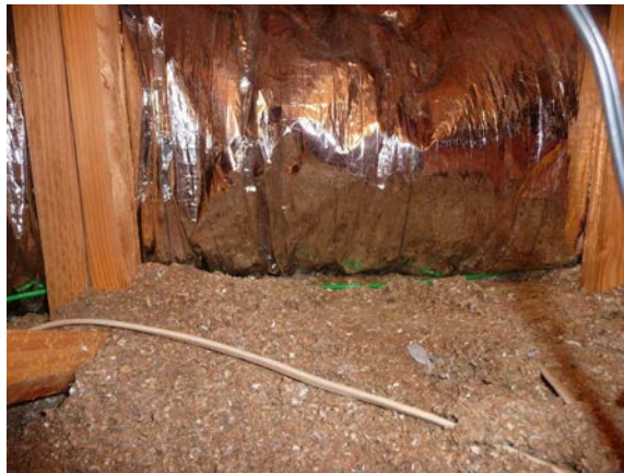
Figure 5. Duct section PA located about three feet downstream of supply plenum prior to insulation
