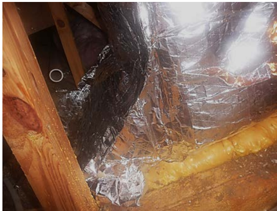
Figure 7. A supply plenum box after insulation wrap was applied. Insulation seams were sealed with reinforced metal tape applied with a squeegee.
