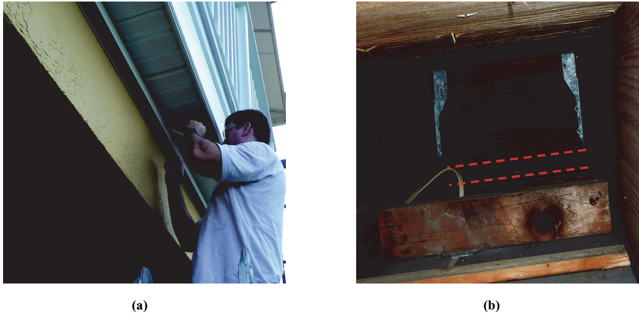
Figure 2 (a) Sections of vented soffit were removed to inspect floor cavities not accessible from attic space. (b) View within cavity sections found pathways about 0.05 m (2 in.) high under floor joist supports that connect to small attic space beyond.
