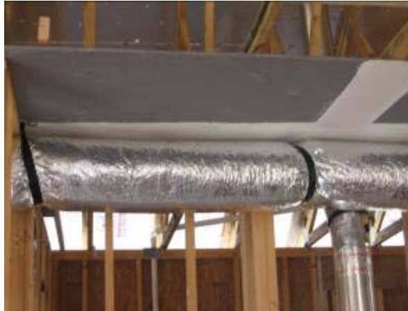
Figure 22. Duct strapped in place prior to finishing the framing of the chase.
