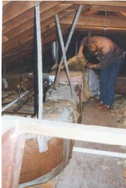
Figure 12. Air handler and duct system installed in a conventional attic. A relatively large volume of air becomes trapped in the system between runtime events, and can encounter significant heat gain/loss to the point where it can cause comfort issues when introduced into the home’s interior.
