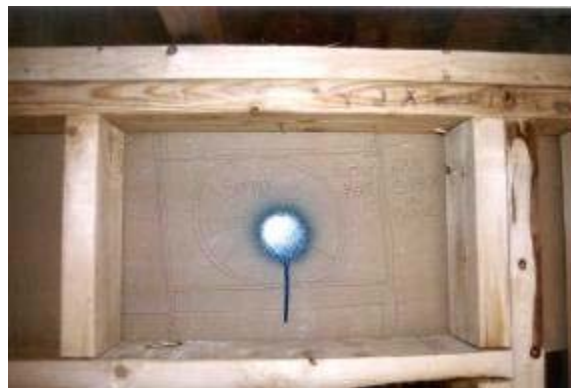
Figure 20. Supply duct location marked in the side of a fur-down chase.
