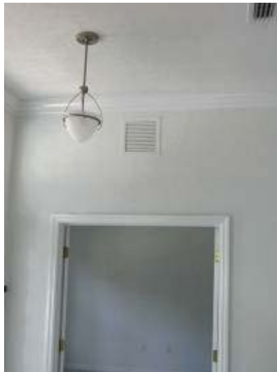
Figure 14. Transom return pathway, through the wall, over doorway of a master bedroom.
