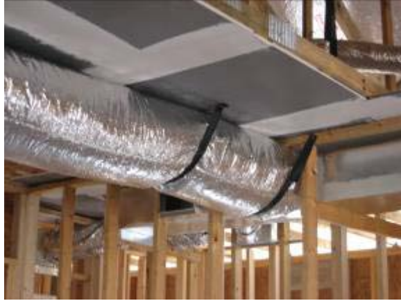
Figure 27. Duct work hung with 2" strapping after chase ceiling drywall installed and sealed.
