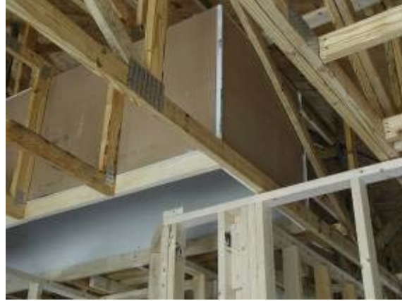
Figure 6. Modified truss work necessitated by fur-up chase.
