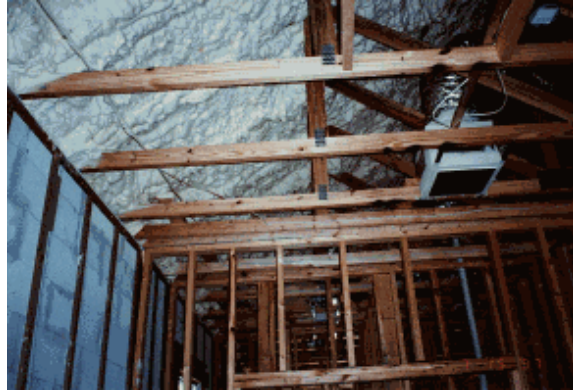
Figure 3. An unvented attic constructed by air sealing the roof deck with foam insulation. Note how the attic duct is now within the home's air and thermal barrier
