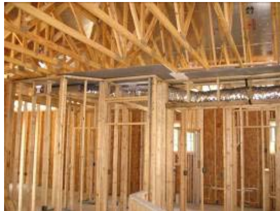
Figure 26. Ceiling drywall installed at fur-down chase top. Drywall is slid through a \frac{3}{4} " + gap between the wall top plate and the truss bottom chord, ensuring a good air barrier.
