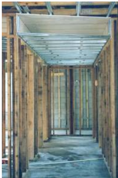
Figure 10. Fur-down chase in hallway. Note the restricted space for the chase due to the 8 ft ceiling height. Note the space-saving, light gauge metal framing at the bottom of the chase.
