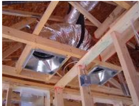
Figure 13. A jump duct through the attic. This will provide return air, over the interior wall. Note this is not an interior duct unless the attic is sealed.
