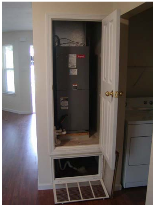
Figure 9. Air Handler Closet
