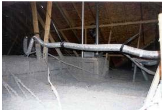
Figure 5. Poorly insulated fur-up chase sides.
