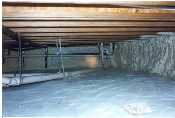
Figure 4. A sealed crawlspace by air sealing the foundation walls with foam insulation.
