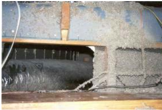
Figure 7. Fur-up chase deliberately used for wiring runs. Also note the poor overall insulation of the chase.
