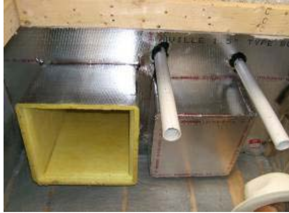
Figure 21. Air handler closet ceiling constructed with duct board.
