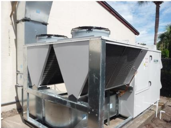
Figure 1. Exterior view of a new VC DX-DOAS located outside a high school cafeteria.
