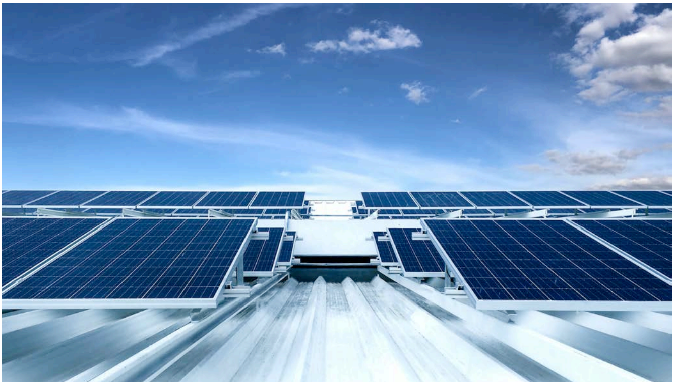
A Solar-Ready Zone is defined and includes new provisions.
