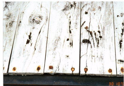
Figure 9 Paint peeling off
