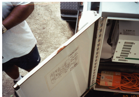
Figure 7 Rust on cabinet doors on Puerto Rico unit
