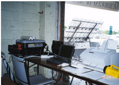
Figure 17 Office equipment powered by PV
