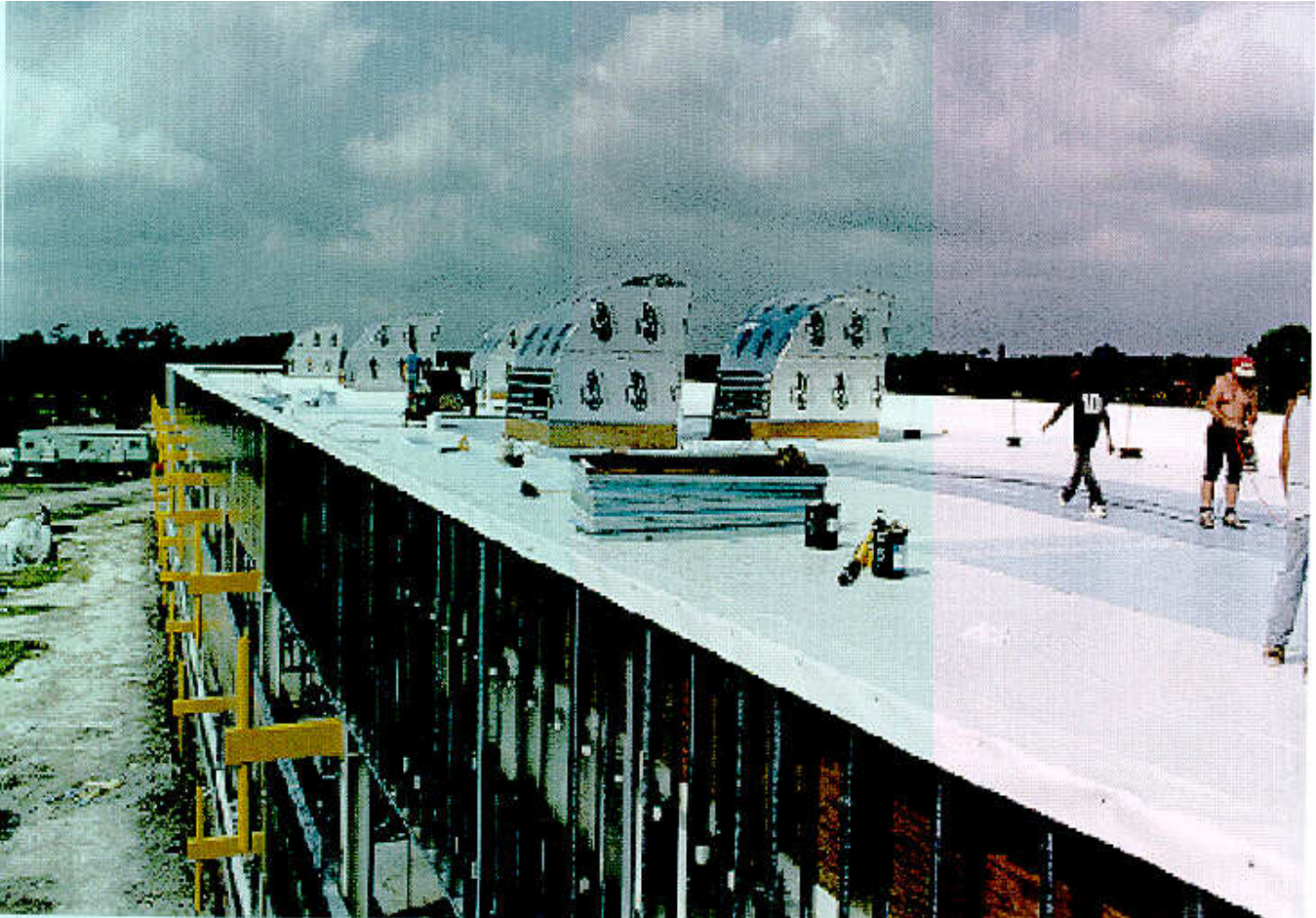
Figure 6: Workers roll out the reflective single-ply roofing membrane (solar reflectance - 70%) over rigid insulation on a metal roof deck. The reflective roof is predicted to reduce building energy use by 4% at virtually no incremental cost. The daylighting roof monitors are clearly visible. These are used to project light into the interior core of the building.
