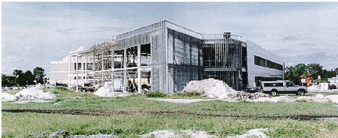
Figure 2: FSEC's new Energy Center under construction in October, 1994. The $6-million facility is slated for completion in late summer of 1995.
