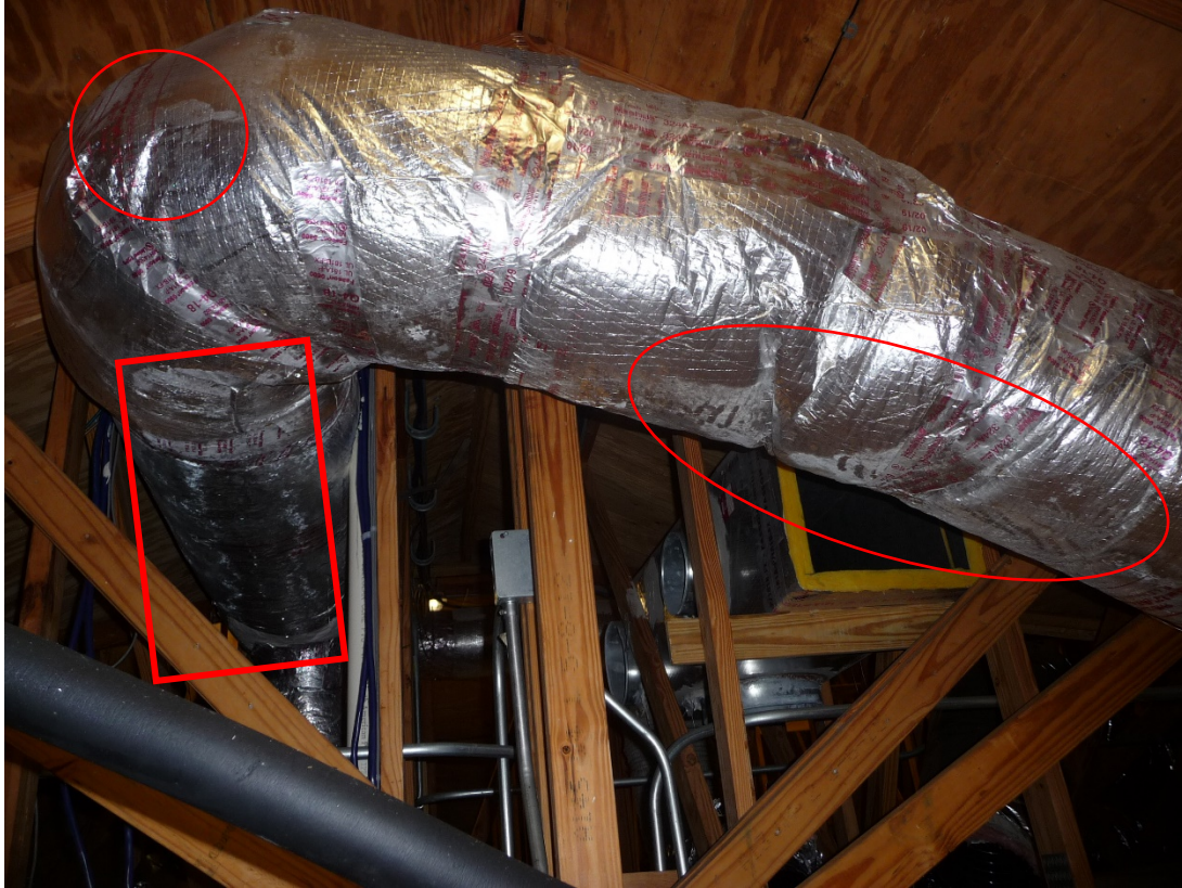
Figure 17. Main trunk section T1 shows light condensation on bottom and some sides (red circles). Heavier condensation and water marking is on the bottom of T1 after bend on left side of photo circles by red rectangle. Photo taken September 18, 2020.
