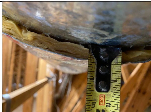
Figure 10. At bottom of T2 trunk line where water was found trapped between duct and insulation.
