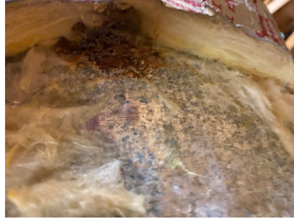
Figure 12. Another close-up view of corrosion spot at T2.
