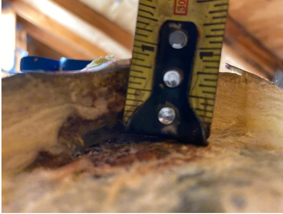
Figure 11. Topside insulation (left side of sample) was about \frac{3}{4} " thick near the corrosion spot.
