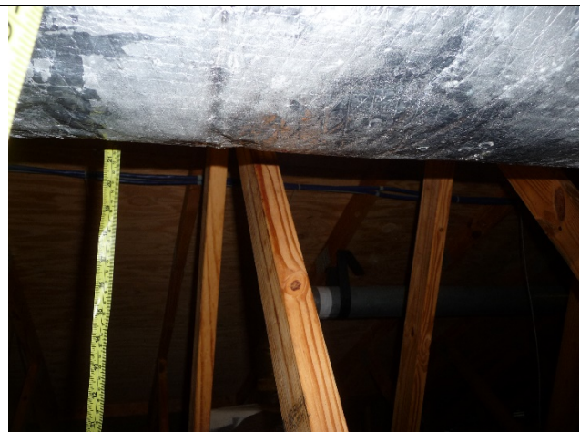
Figure 21. Condensation and water drops on bottom of main trunk T3 (9/18/20).
