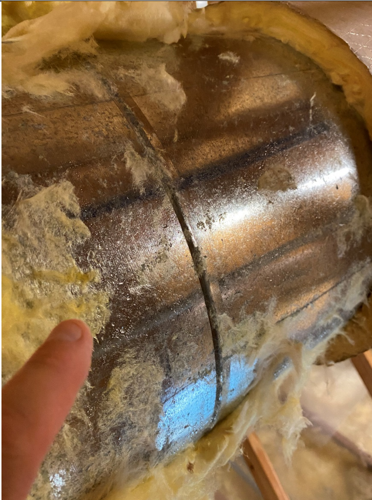
Figure 13. Water droplets observed on metal duct T2 immediately after pulling away insulation sample.
