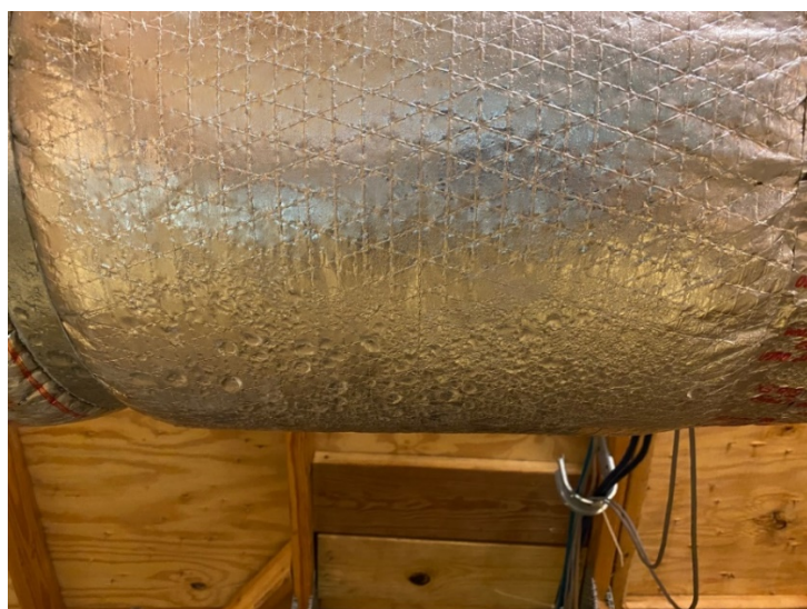
Figure 1. Significant water condensation on exterior insulation jacket wrapped around an airtight metal duct supply system in a vented attic August 24, 2020.
