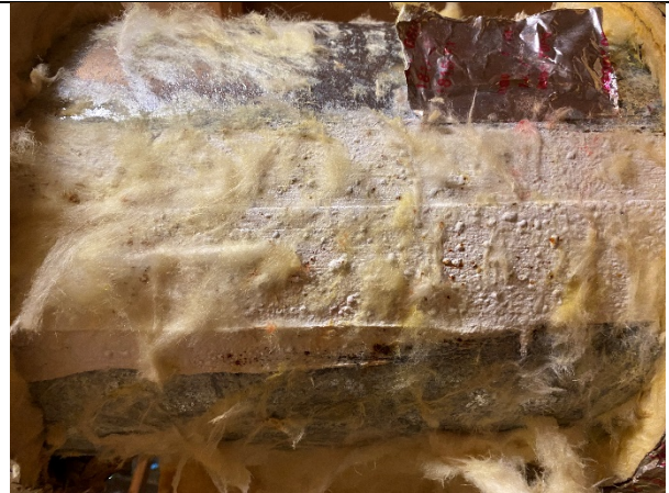
Figure 15. Close inspection at the T3 sample found water droplets near top and on bottom of the metal duct. Corrosion can be seen at the mastic duct seam on metal duct.
