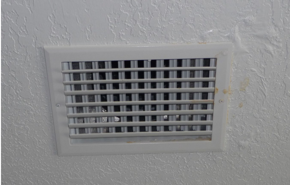
Figure 16. supply grille on duct branch B1 has visible water on grille and staining and paint damage on right side. The integrity of the drywall was still good. Photo taken September 18, 2020.
