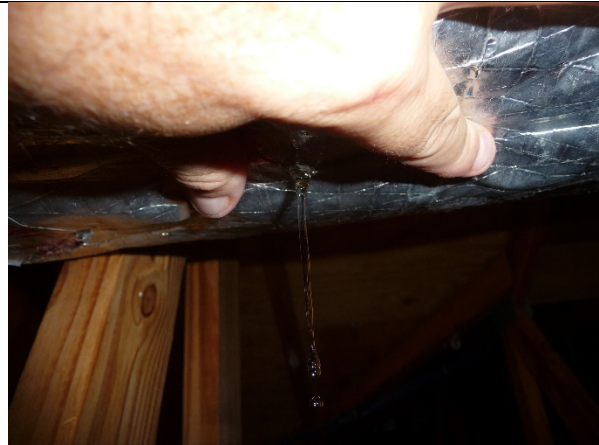
Figure 23. A steady stream of water can be seen coming out of the inspection hole in jacket while applying pressure on jacket. Water was trapped inside jacket throughout the main trunks.
