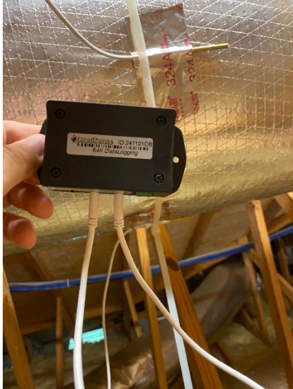
Figure B2. Temperature and RH sensor logger used on and around ducts in attic.
