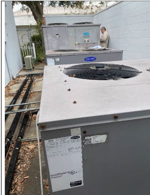
Three condensing units serving for AC1 and AC2 are in decent condition.
