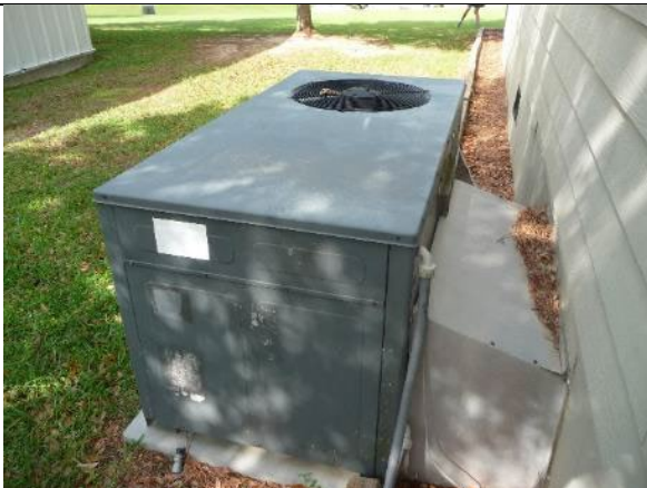
Old package air conditioner at MI-1 office.
