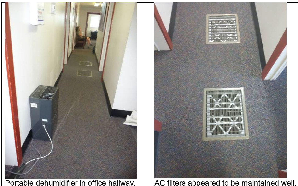
Figure 36. MI-1 office package unit, thermostat, portable dehumidifier, and air distribution filters.
