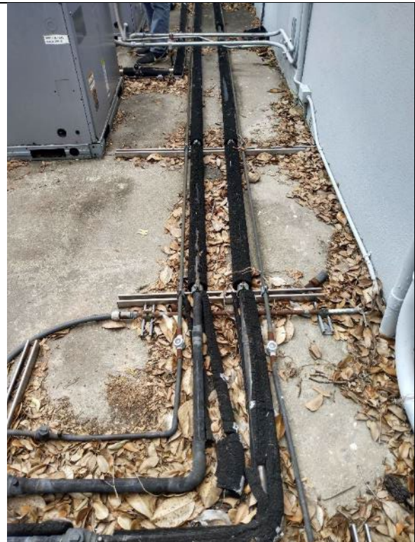
Refrigerant lines show advanced degradation of insulation and some parts of copper pipe such as near the site glasses.
