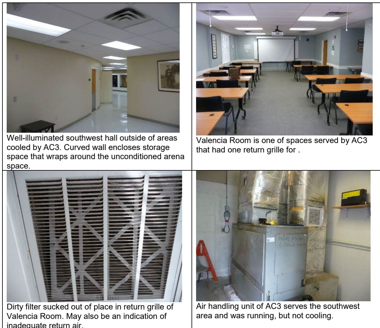
Figure 18. Example interior lighting and HVAC images.
