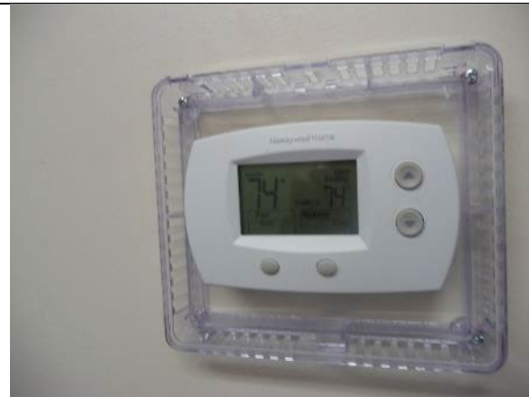
The AC cooling setpoint was observed at 74F.
