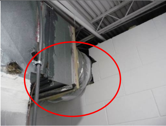
Figure 10. The main supply duct trunk serving the east building is severely constricted.
