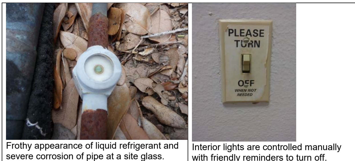
Figure 21. Condensing units, degraded refrigerant lines, and manual lighting control.
