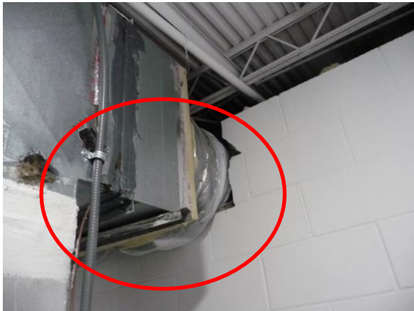
Figure 5. The main supply duct trunk serving the east building is severely constricted.
