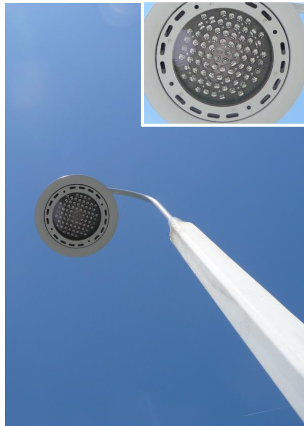
Exterior LED light is about 50% to 90% more efficient than HID lamps and should last about 4 to 8 times longer. Photo: Charles Withers Jr.
